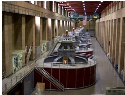
Figure 20.43 Hydroelectric generators at the Hoover dam. (credit: Jon Sullivan)
